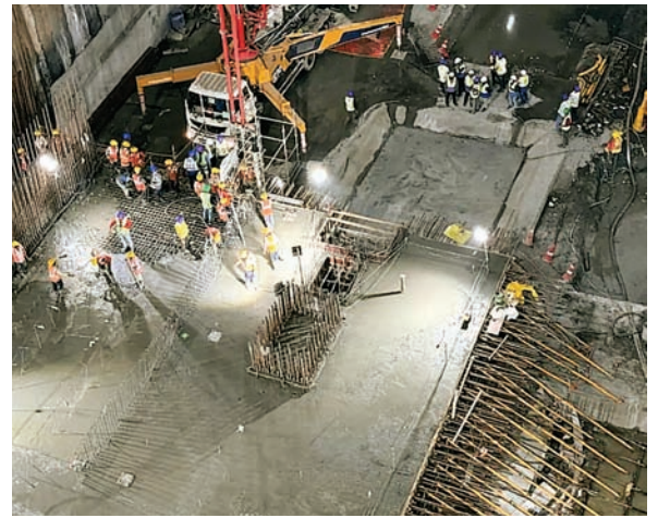
69 slabs that are cast for the station, which will form the deepest construction level for the Bullet Train station.
