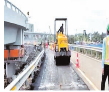
road". It added that the re-patch work on the cracks -- detected at three locations -- has been taken up without disrupting the MTHL traffic. The MMRDA also said that contrary to the rumours, the cracks are not on the MTHL bridge, but on the approach ramp towards Mumbai on the Navi Mumbai end. "The cracks on Ramp 5 are minor longitudinal cracks in the asphalt pavement and do not indicate any structural defects," the MMRDA said. The repair work has been taken up by
