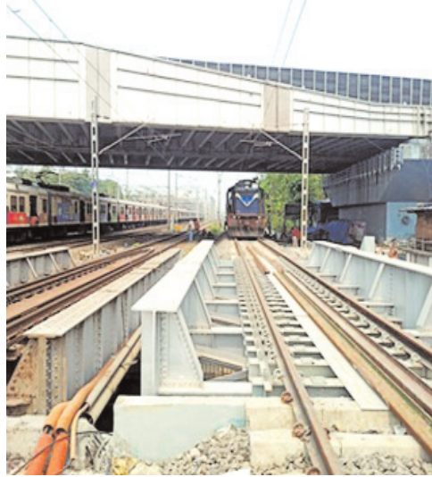
5th and 6th lines has been provided with the Bandra Terminus Yard after slewing of 700-metres existing tracks and dismantling of five points
