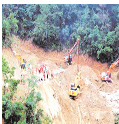
The Ministry of Emergency Management has dispatched a team to the
