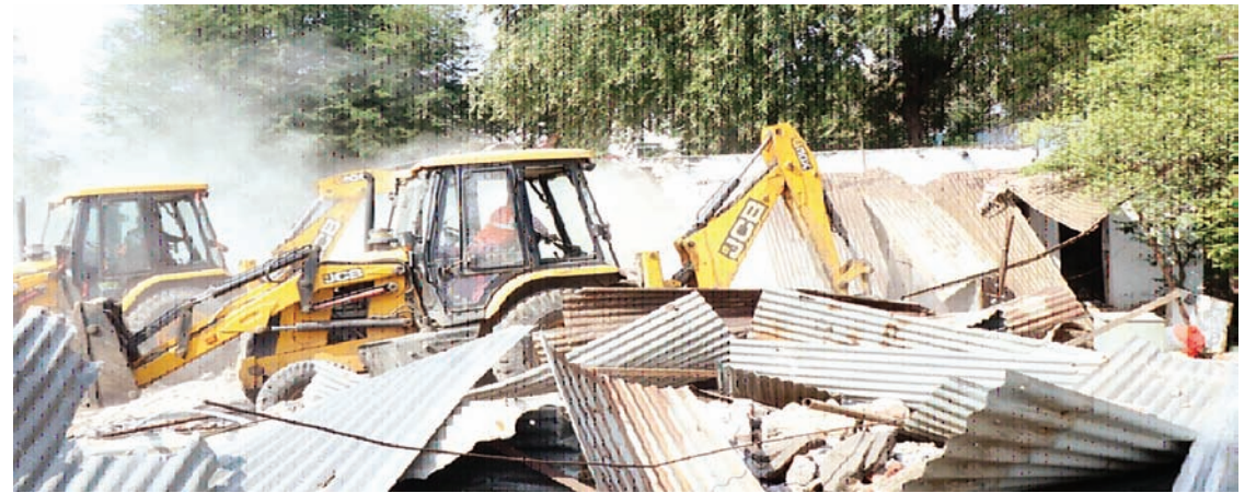
removed the illegal encroachment by running a joint operation. The agricultural farm and tin shed built on the encroached land have been demol-
